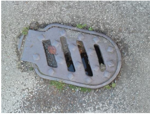
Pipeline access point
