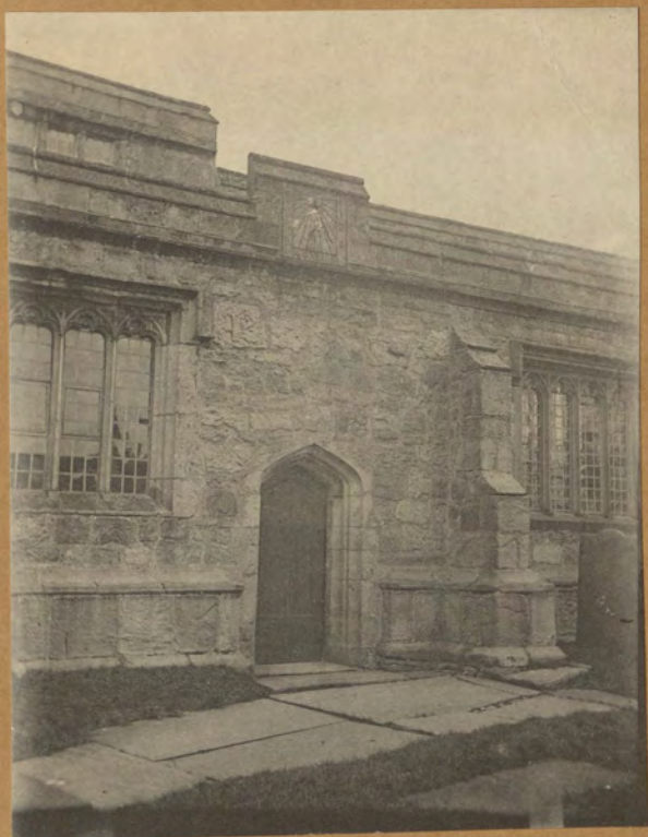
Small South Door of Church, showing sundial and foundation of old buttress.
