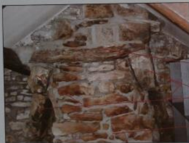
INNER STACK Old fire smoke box Other end of stone corbels New internal chimney stack
