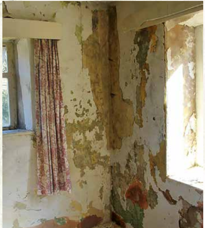
Interior of first floor damp walls before removal of cementitious materials prior to wood fibre insulation and lime plaster
