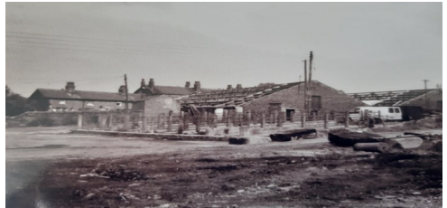
A similar view of the Main Road Front Docks under demolition. 1990's
